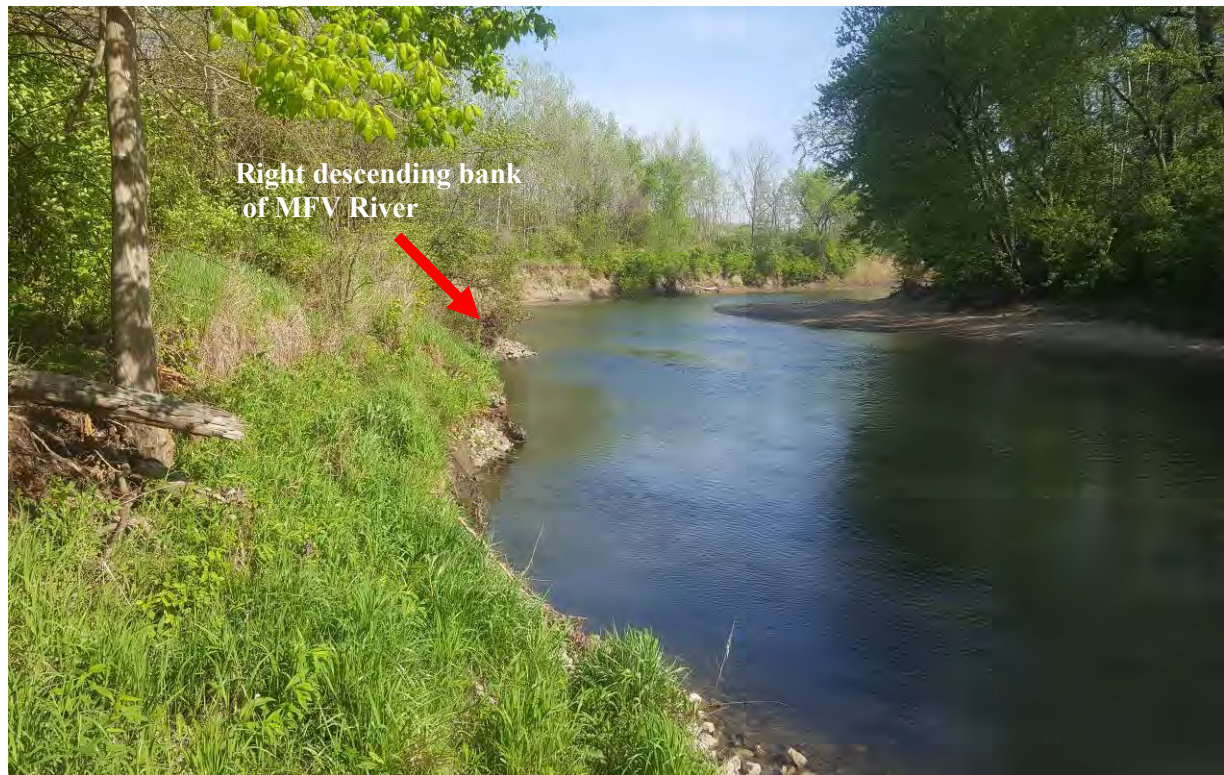
Photo 5. Photo along right descending bank of the river near existing gabion area, facing upstream north (4-26-17)
