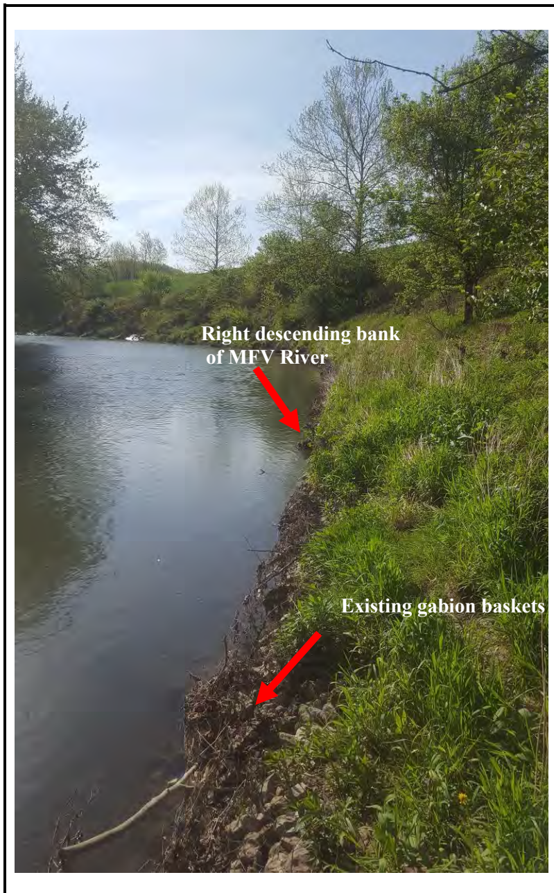
Photo 4. Photo along the right descending bank of the river showing the existing gabion baskets, facing downstream south (4-26-17)
